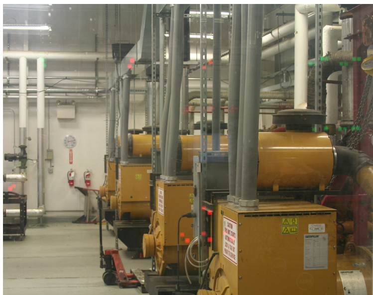
Diesel generators operating inside the Unalakleet Valley Electric Cooperative. Photo: Putt Clark, REACH Up.
