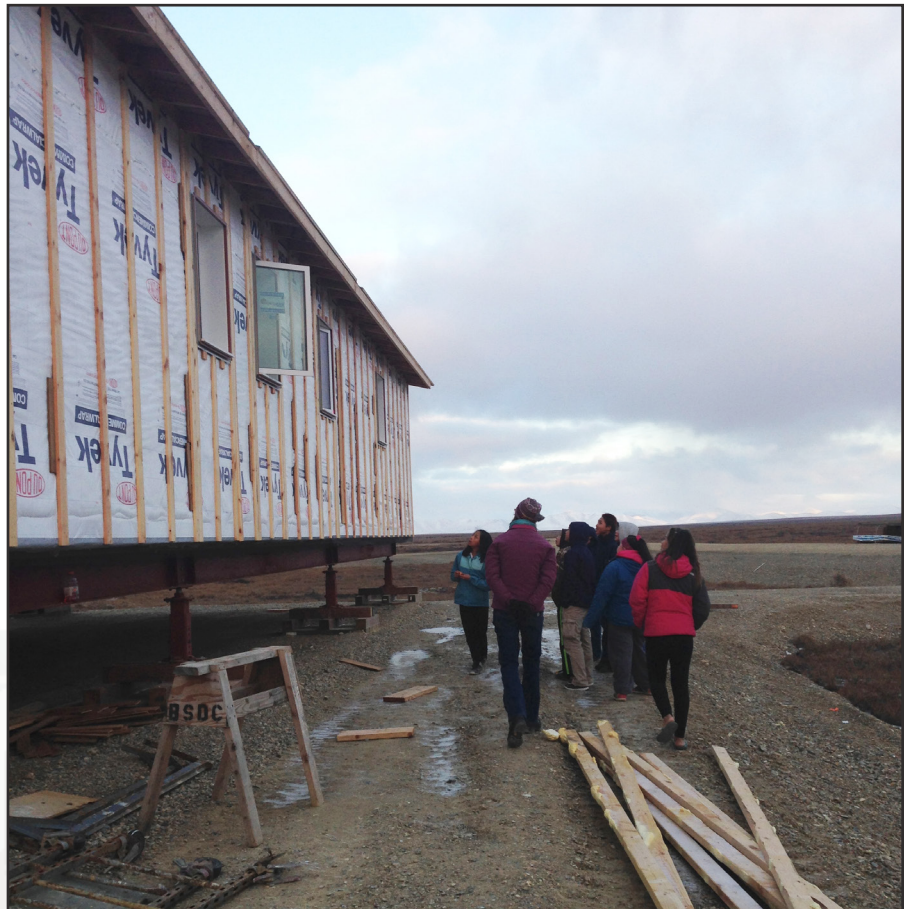
Robbin Garber-Slaght leads students on a tour of a house being built in their village of Brevig Mission. Garber-Slaght is a Product Testing Lab Engineer at the Cold Climate Housing Research Center in Fairbanks. Photo: Sally Kieper, REACH Up.
