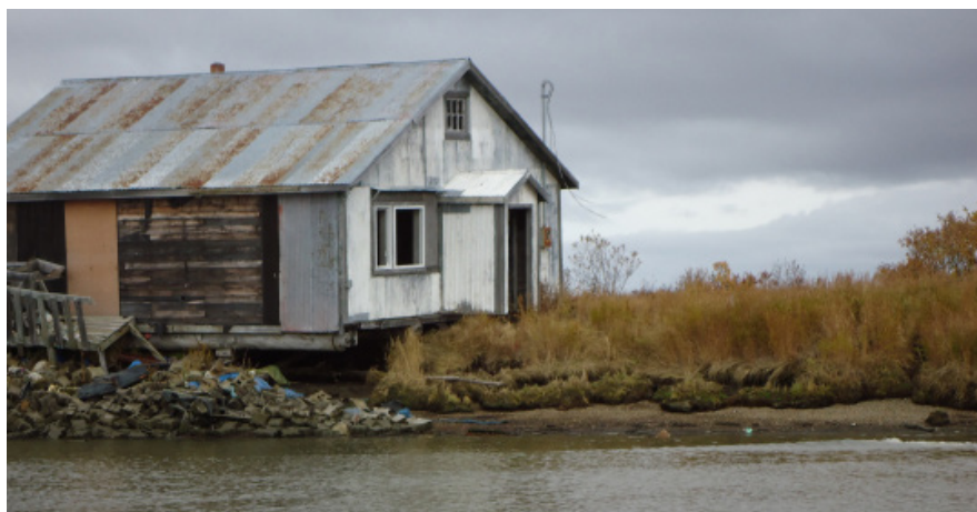
Erosion caused by the movements of the slough in Kotlik.
