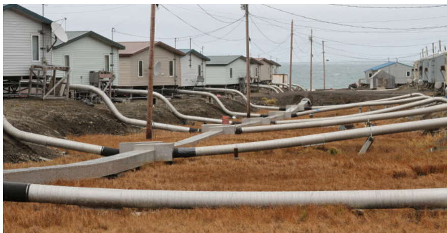
Water lines run over the tundra to houses in the village of Savoonga. Photo: Yuri Bult-Ito, REACH Up.
