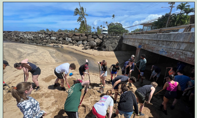
Nome & Wai'anae students, work together to repair a historic fish pond. Photo: K-12 Outreach Staff.
